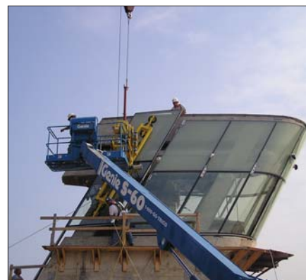
12 vacuum cups lift curved IG unit into place on the tower, powered by U.S. Curtainwalls' proprietary lifter.
