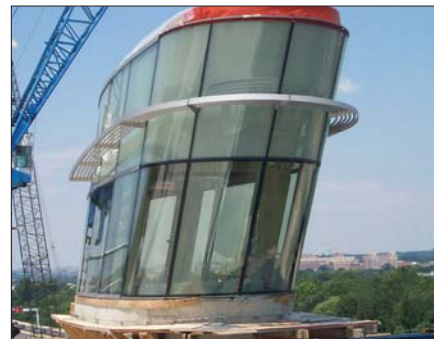
The bent glass trapezoids, sealed with Edgetech's flexible spacer, have virtually no straight lines or 90° corners.
